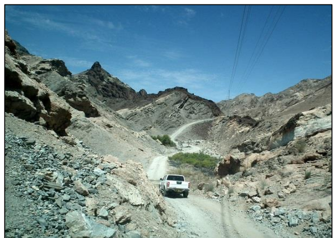
The new Lithops-Husab power line runs through some extremely rugged terrain (photos Ann Scott)
