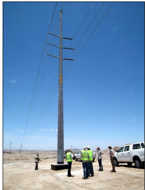
The new Lithops-Husab power line uses a steel-type monopole about 25 m high; the (horizontal) insulators are 1.5 m long
