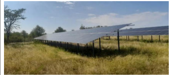
Photo 4-22 Photovoltaic solar system
