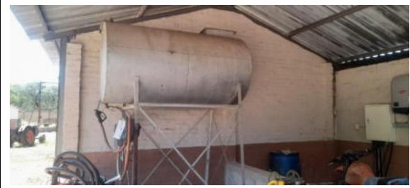
Photo 4-20 Fuel storage tanks
