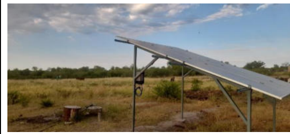
Photo 4-19 Solar panel used at boreholes
