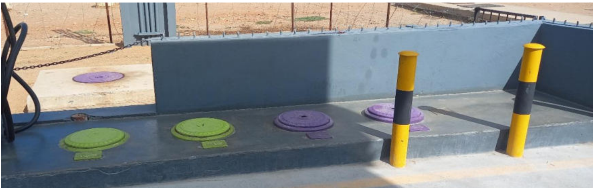
Figure 9: Fuel Receiving Points from Road Tankers
