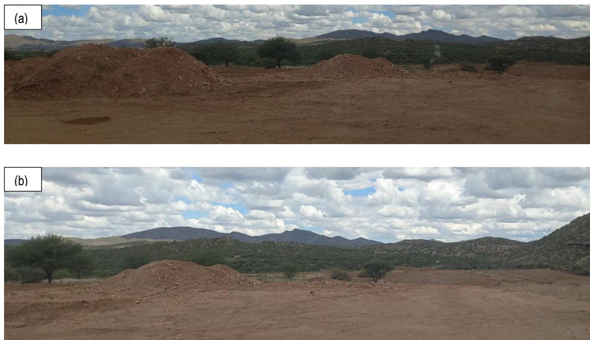
Figure 5: Civil works at the new cemetery (a) & (b) to the east of the gravel extraction site
