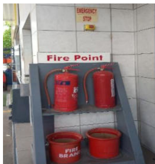
Figure 12: Fire extinguishers & spill cleaning sand
