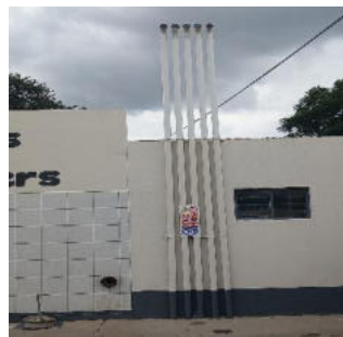
Figure 7: Vent pipes from the tanks
