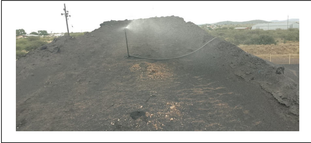
e) water sprinklers installed on the waste charcoal fines
