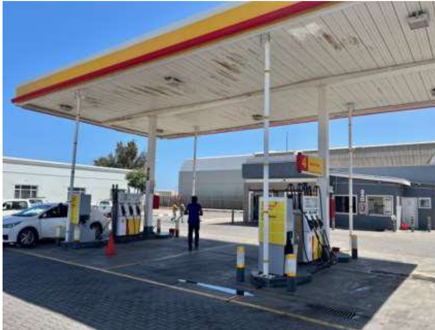
Photo 1. Fuel installation at the site
