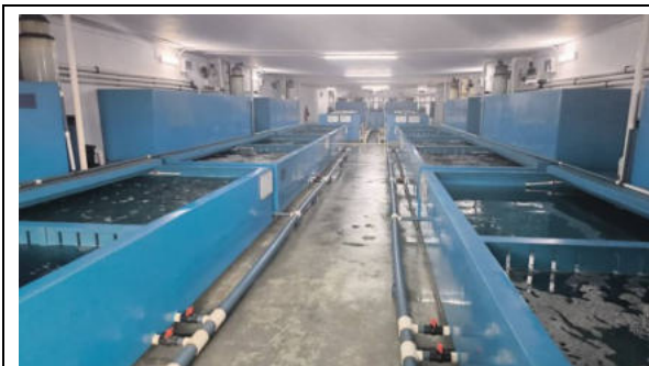
Photo 4-7 Holding tanks at the processing plant
