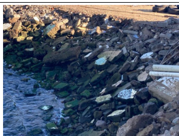
Photo 4-12 Seawater discharge point
