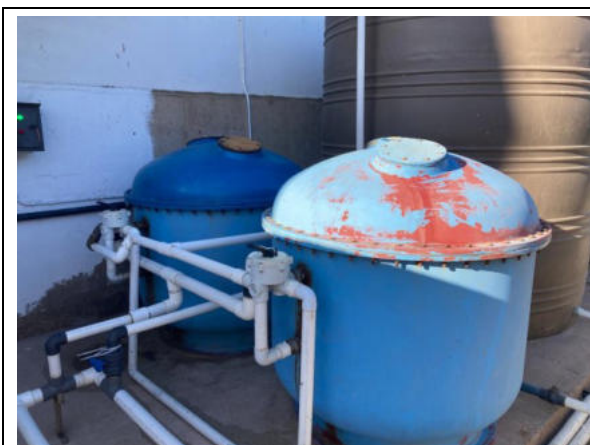
Photo 4-9 Sand filters used for water filtration
