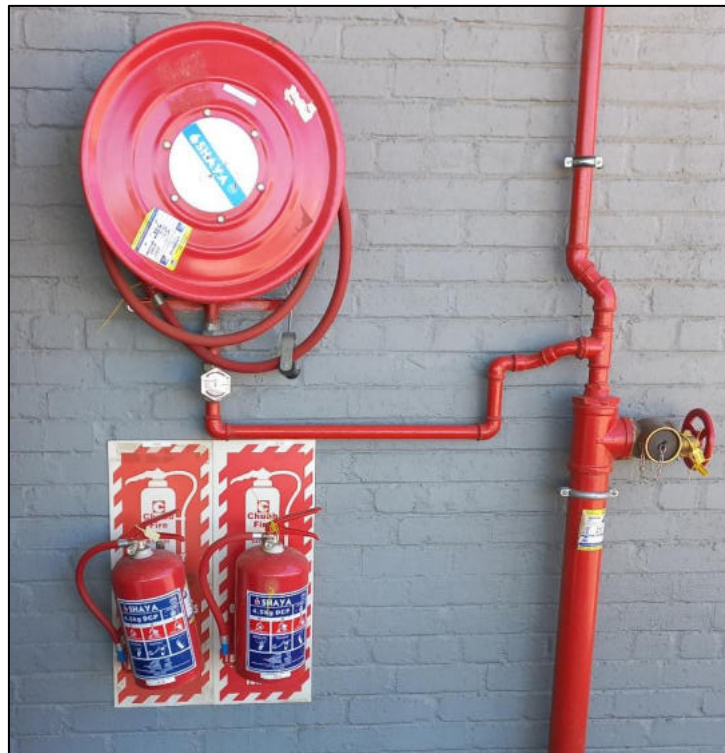
Figure 12: One of the fire extinguishers on site
