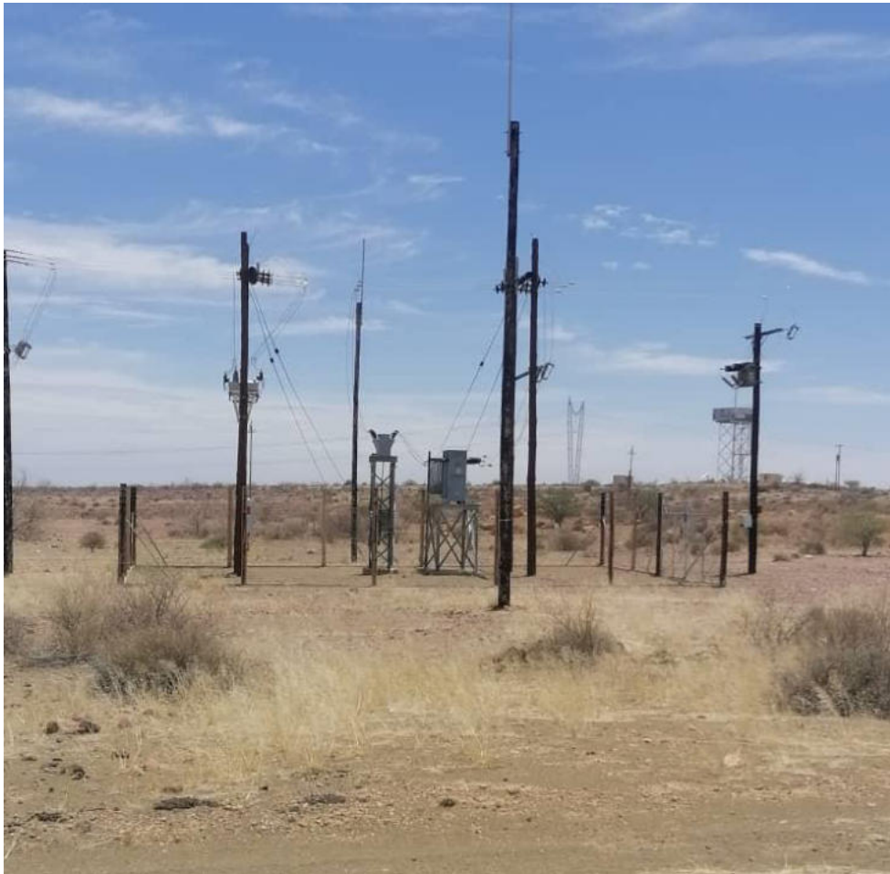
Figure 6: Sub-station and powerlines opposite the proposed site
