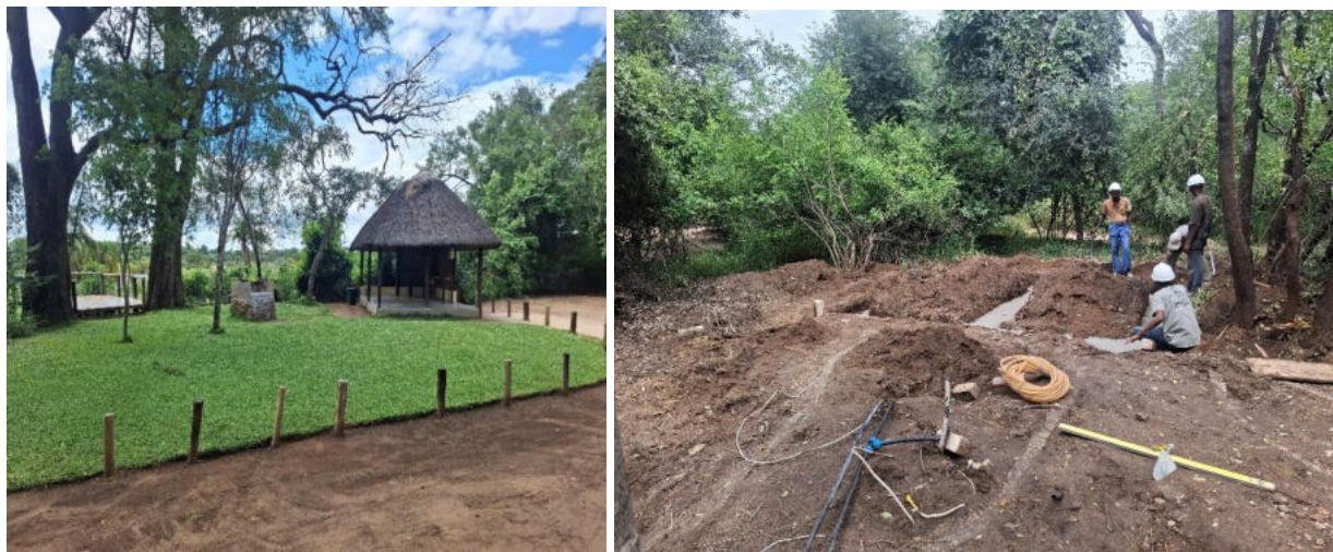
Figure 20: Campsite No. 1 is currently being reconstructed to a VIP campsite (new ablution facility).
