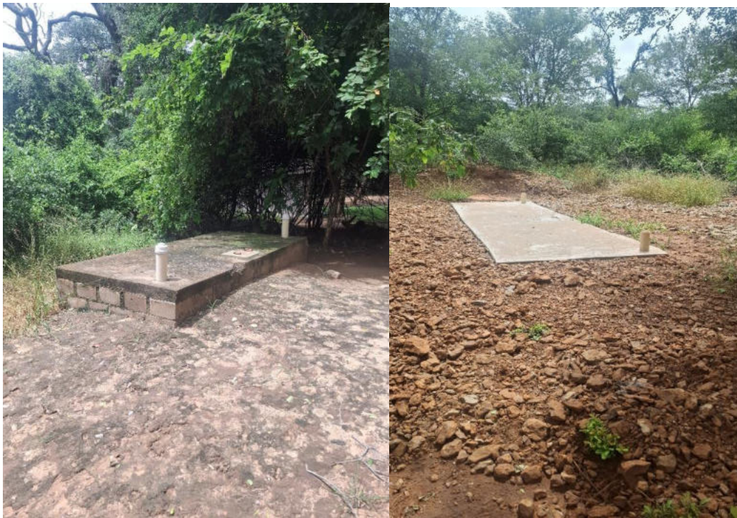
Figure 13: Stage 1: Two-chamber septic tanks at Campsite 6-9 with 8000- liter capacity (LHS) and Luxury rooms with 10000- liter capacity (RHS) emptied and transported to Stage 2
