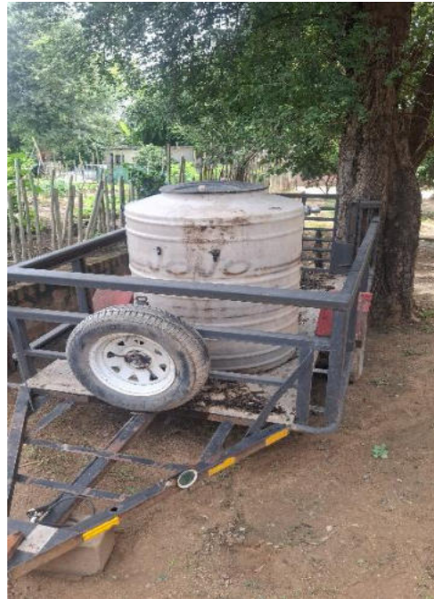
Figure 17: The trailer used to suck up effluent from Stage 1 septic tanks and transport the effluent to the Stage 2 digester system
