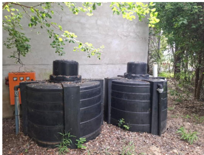
Figure 14: Stage 1: Two separate plastic septic tanks at main restaurant pumped directly to Stage 2 (5 x Chalet septic tanks are also fed directly to this system)
