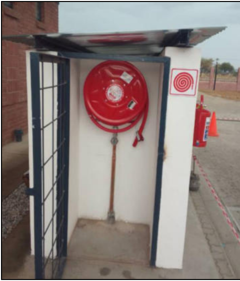
Figure 15: Fire protection equipment
