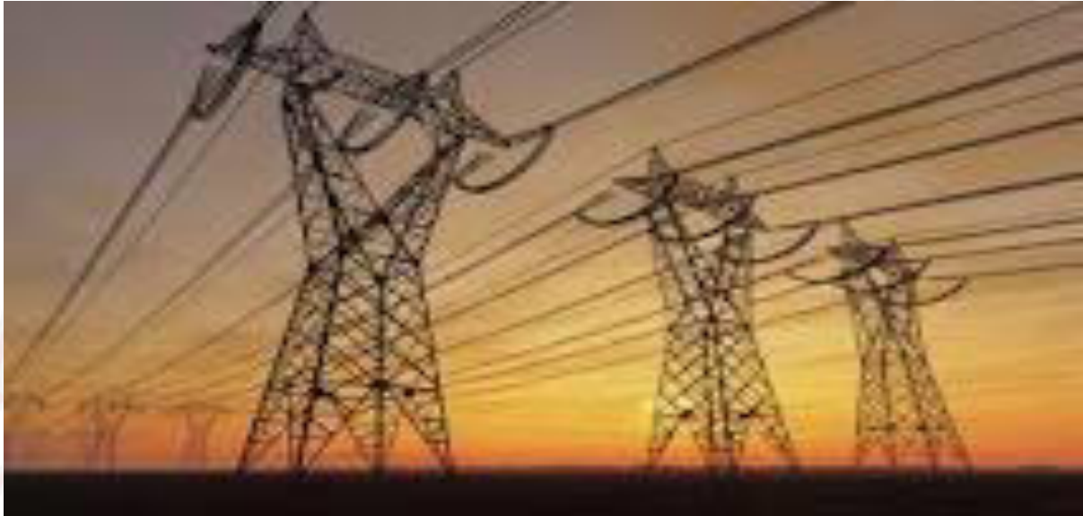
Overhead power lines at Maposa Area
