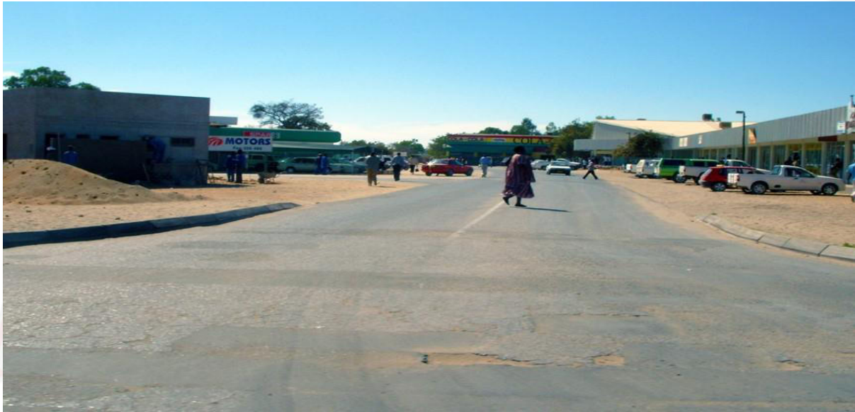
Picture showing road with pothole patches and potholes in Rundu
