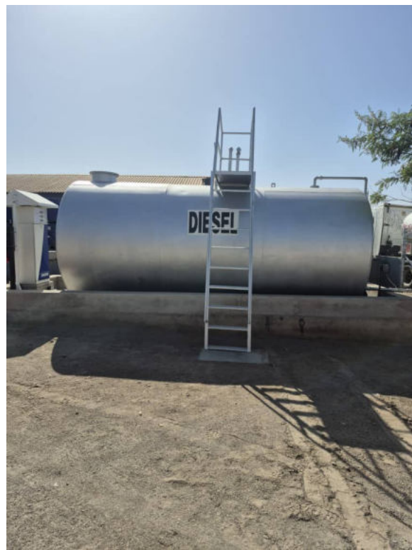
Photo 4-1 Diesel storage tank in bund area
