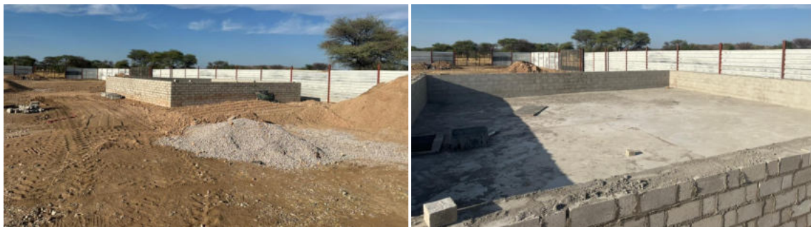
Figure 5. Fuel Tank Platform and 110% spill containment wall
