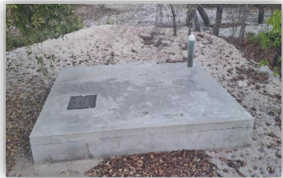
Newer Septic Tanks
