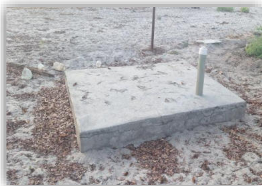
Older Septic Tanks
