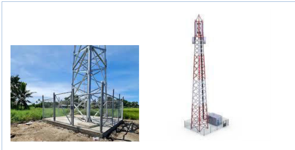
Figure 2: Typical lattice tower (for visual purposes only)
