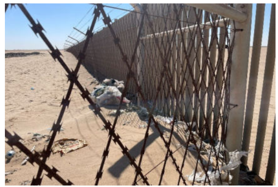
Photo 3-14 Windblown waste caught in the boundary fence
