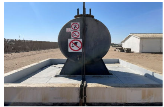
Photo 3-12 Diesel tank for backup generators
