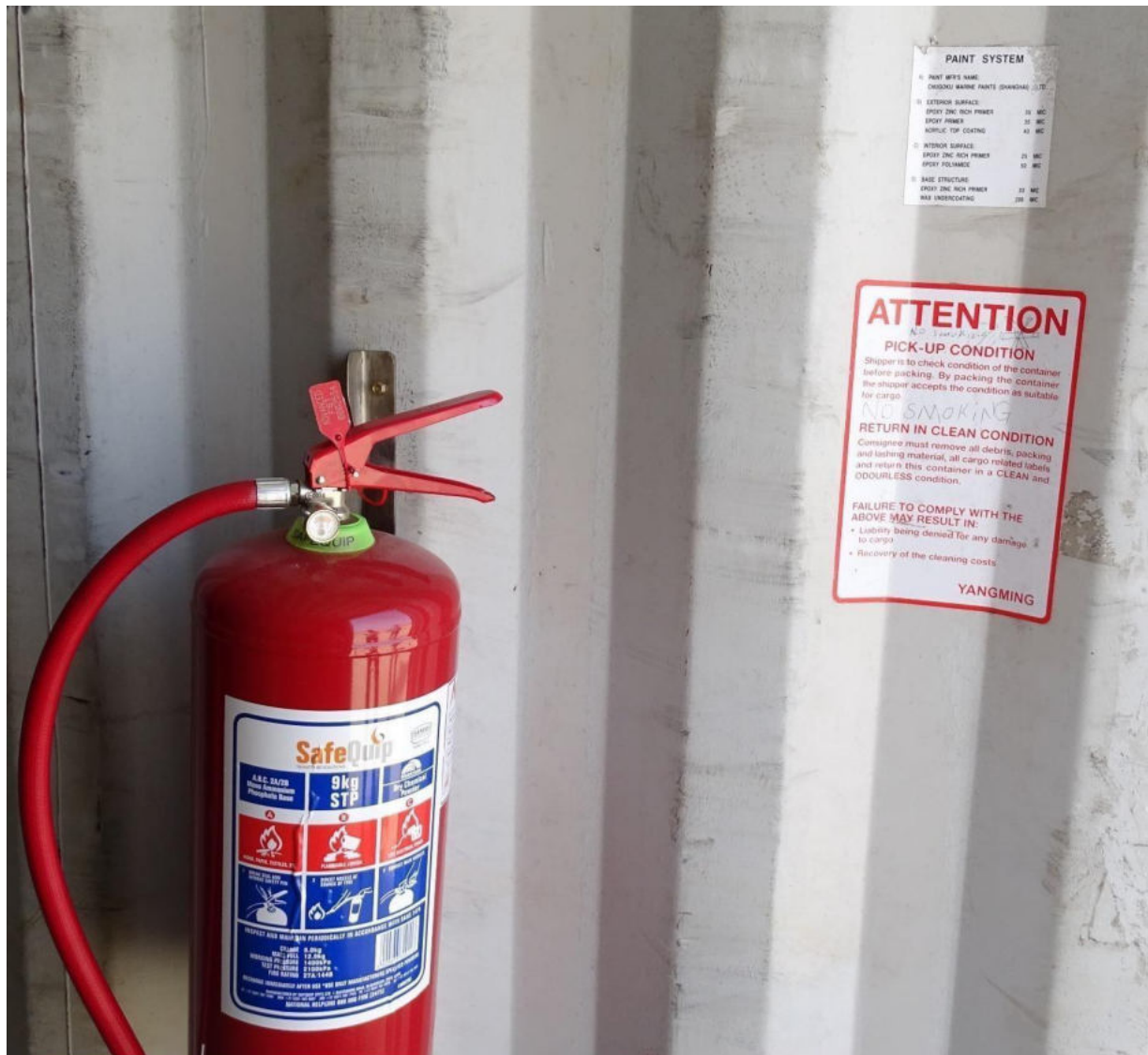
Photo 8, Fire extinguisher in the oil storage shed for fire fighting response and awareness precaution.
