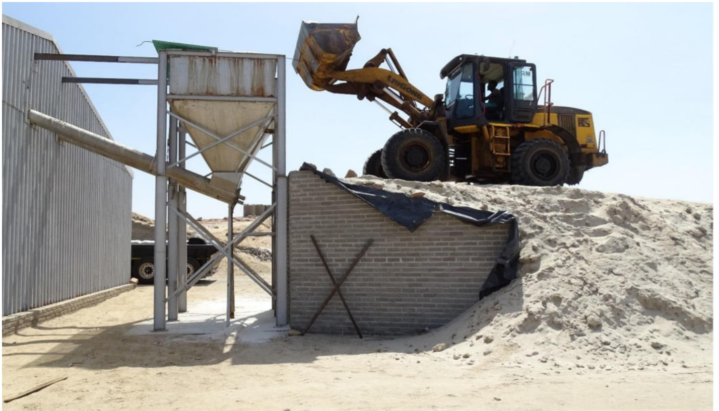
Photo 14: Latest Visual changes to the newly fully commissioned coarse salt feed ramp to the hoppers
