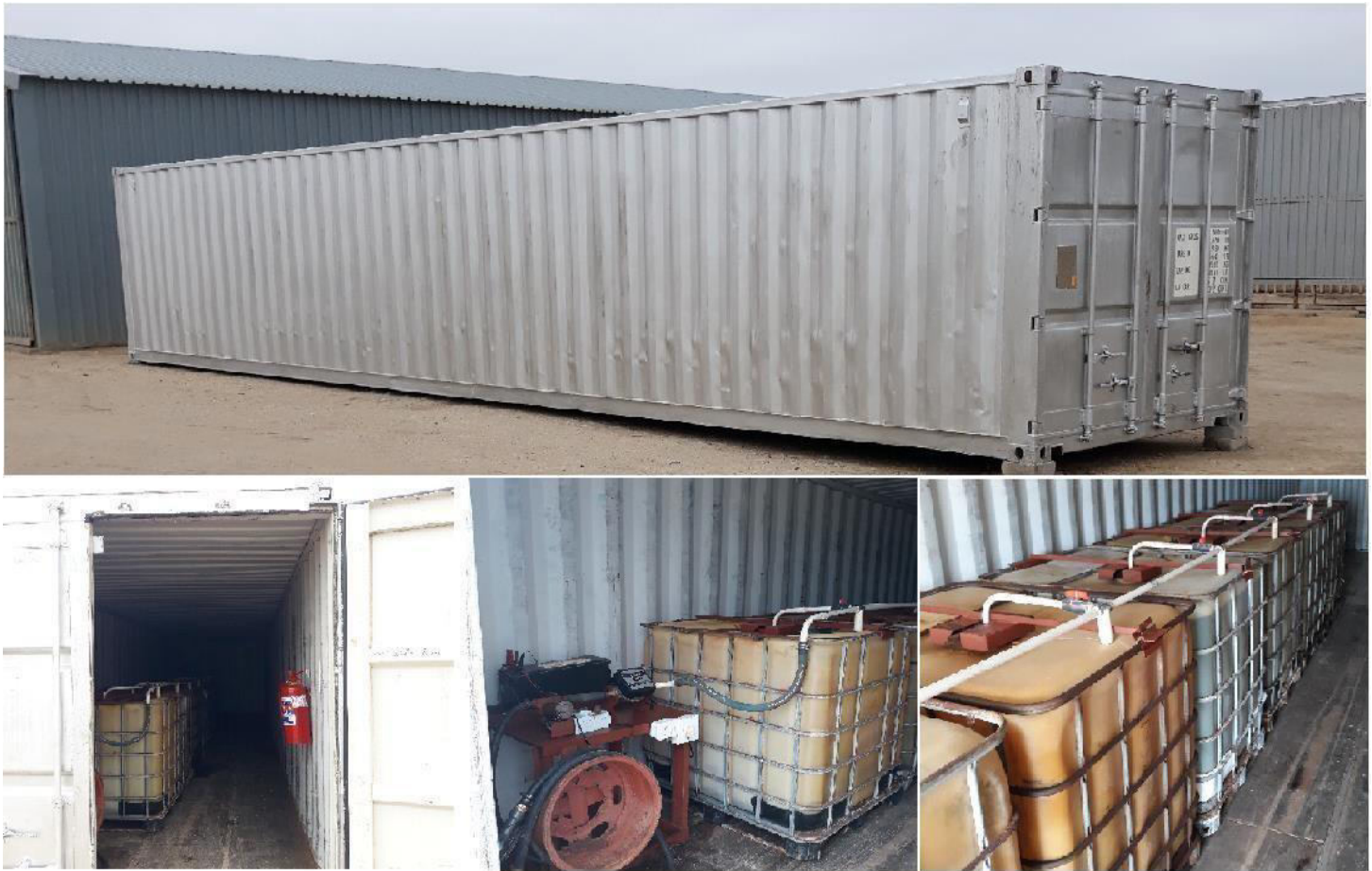
Photo 13, latest photos of the latest installed petroleum storage and dispensing facility.
