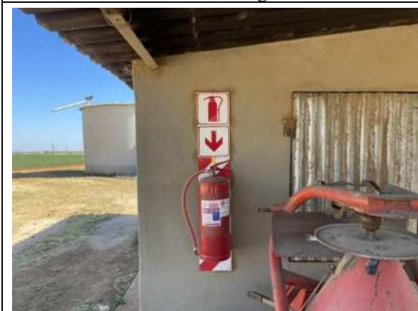
Photo 4-33 Fire extinguisher post
