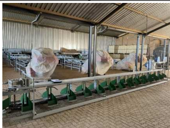
Photo 4-12 Potato bagging station
