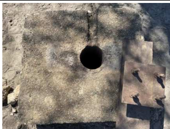
Photo 4-45 EB 6 Not used/collapsed borehole
