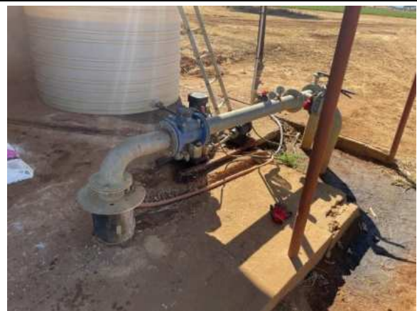
Photo 4-40 EB2 / WW204677 Irrigation-use borehole
