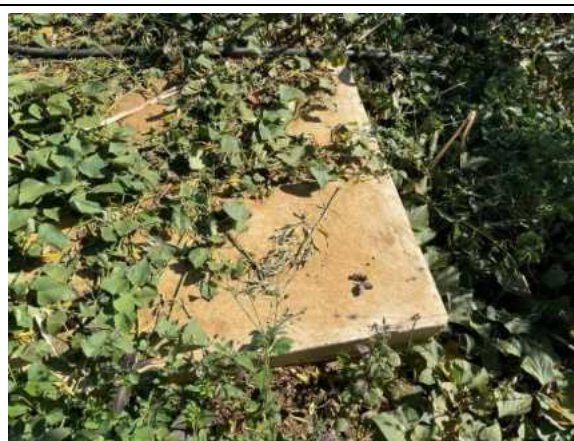
Photo 4-48 Septic tank at worker housing
