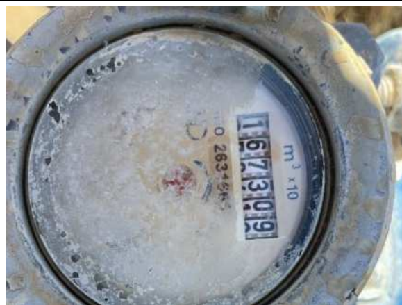
Photo 4-43 Flow meter on EB4
