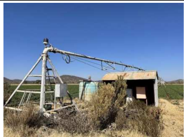
Photo 4-38 Centre pivot base
