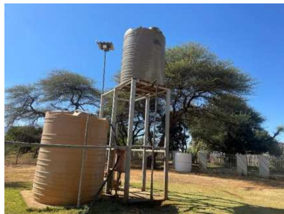
Photo 4-25 Raised domestic water reservoir
