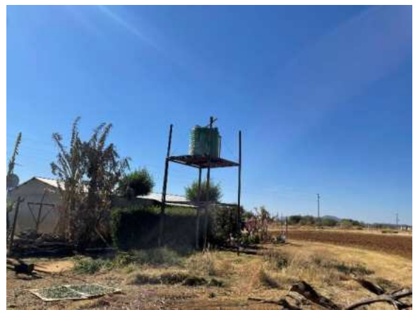
Photo 4-26 Employee water reservoir
