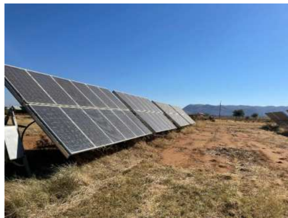
Photo 4-21 Photovoltaic solar installation
