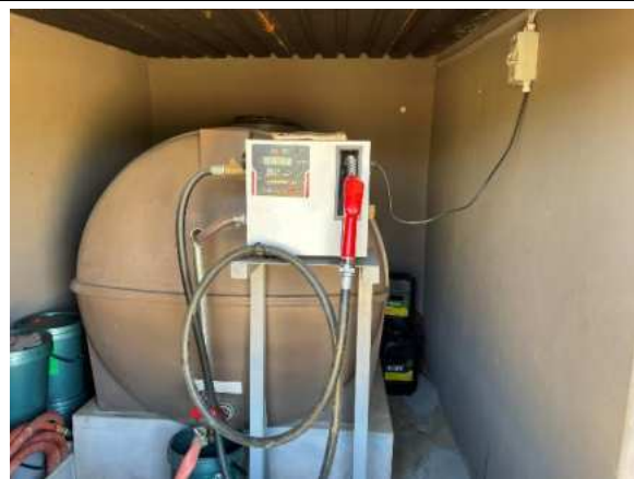
Photo 4-23 Fuel storage tank
