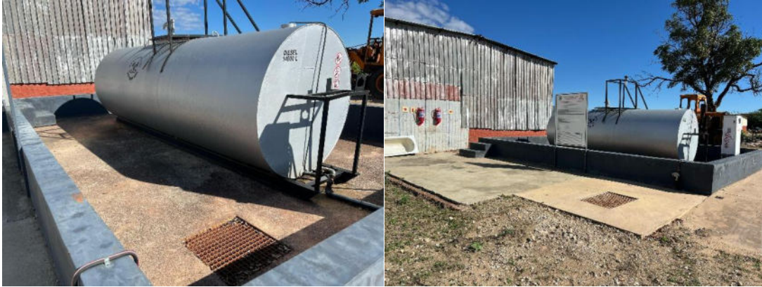
Figure 2-5: The 14,000-litre diesel tank onsite
