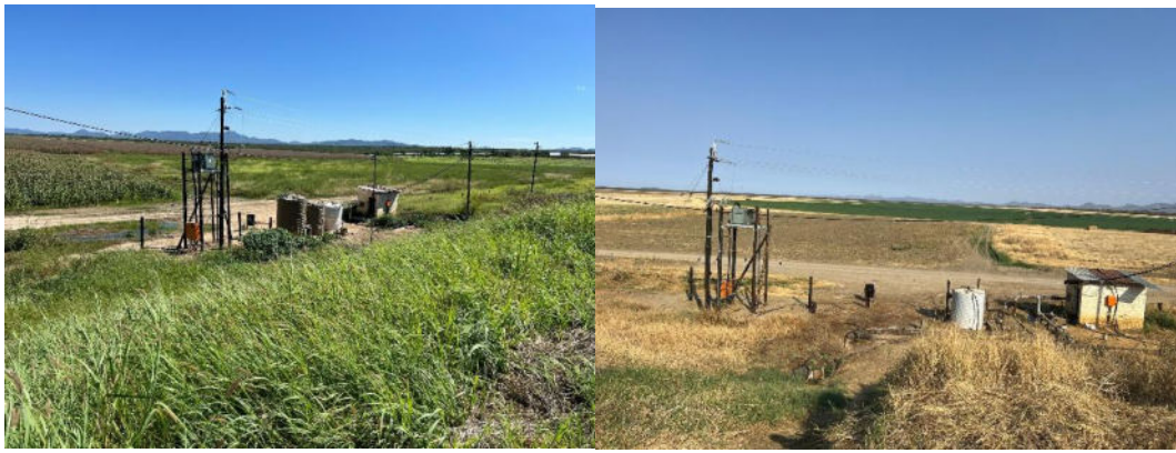
Figure 2-3: The CENORED powerline on the Farm
