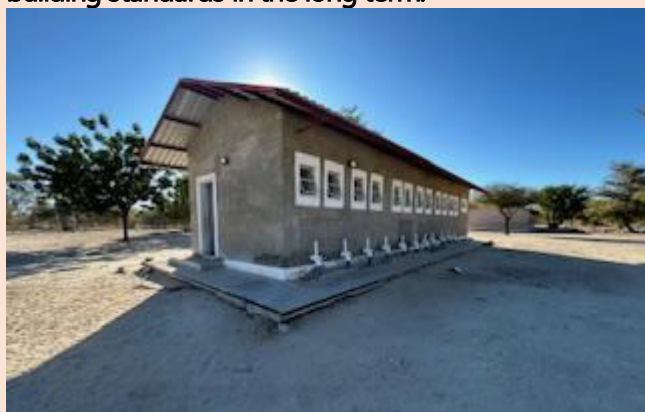
Sharp apron edges (fix and land fill).
