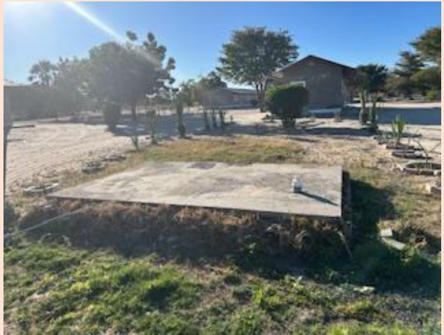
Septic Tank No. 1: (Empty and close it urgently )
