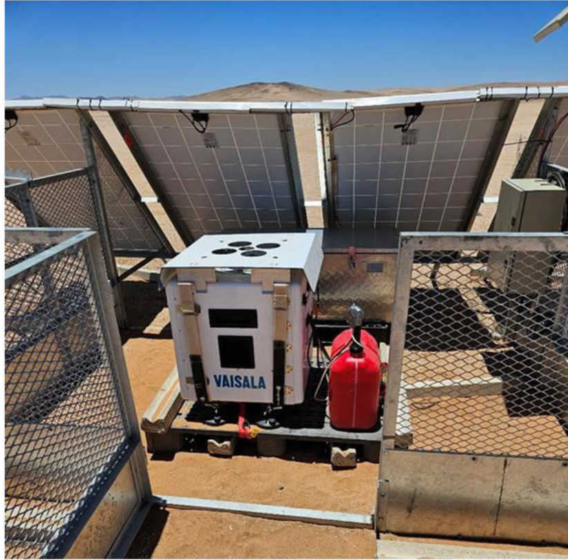
Figure 2-3: Example of LiDAR Installation (Option 1) for PML04 (source: GEO-NET, 2025)
