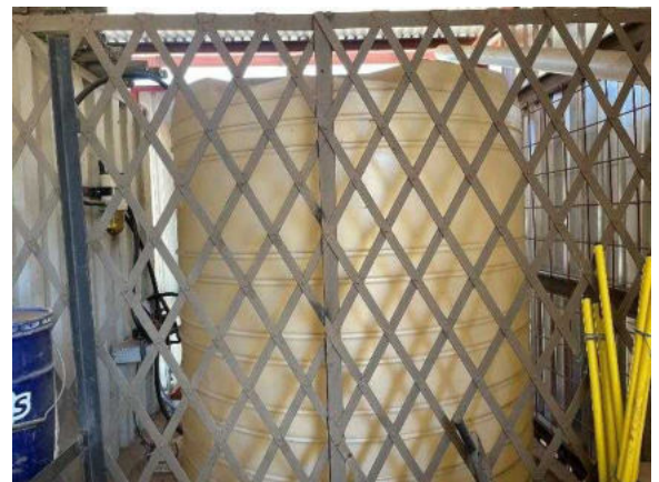
Photo 4-16 Fuel storage tank
