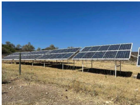
Photo 4-15 Solar installation used at boreholes
