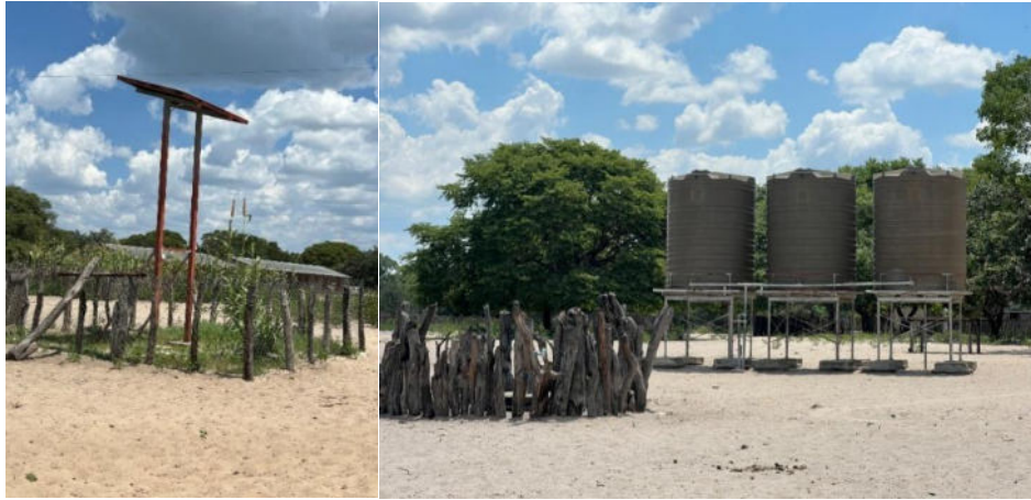
Figure 5-6: The community solar panel and water tanks in Shanyashi
