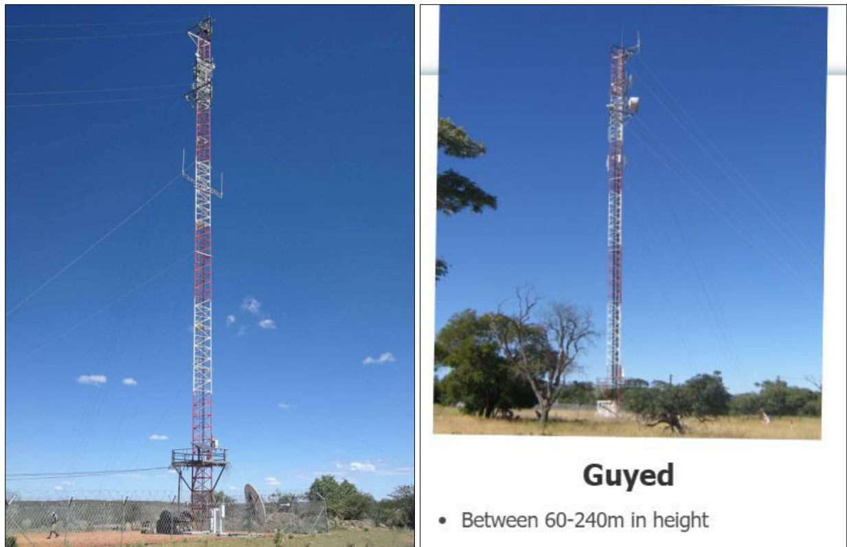
Figure 2-1: Typical red and white painted guyed mast tower structures in Namibia (source: MTC Namibia and https://powercom.na/ )
