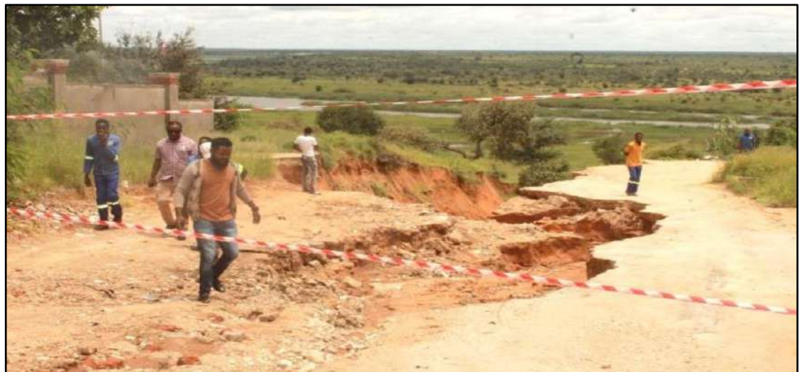
Figure 13: Erosion - Access Road Damaged by Storm Water
