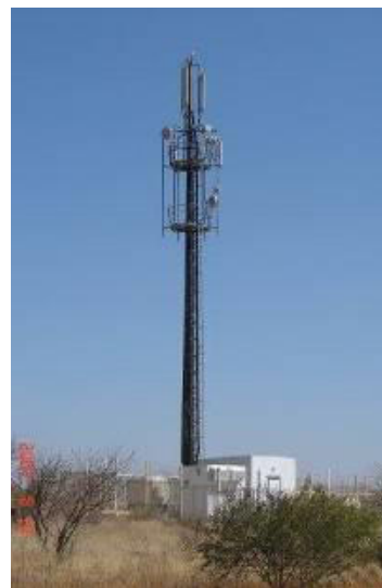
Figure 5-4: Example of BTS (Monopole)
