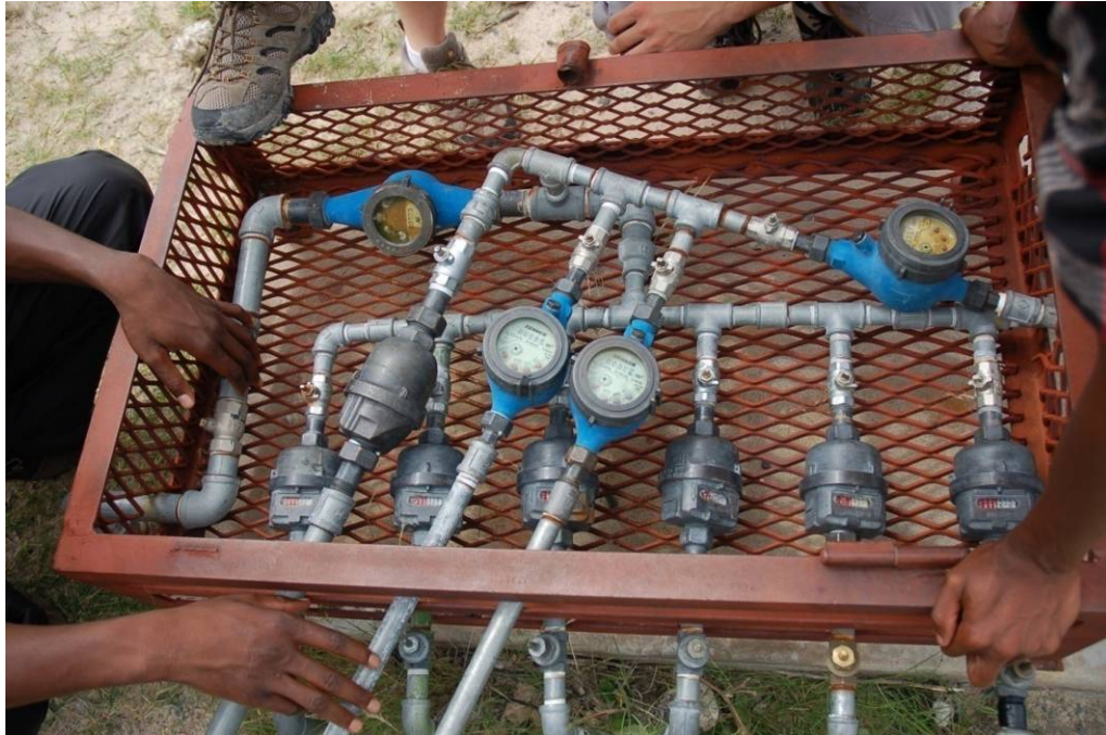
Water point water meters, used by NamWater for water billing
