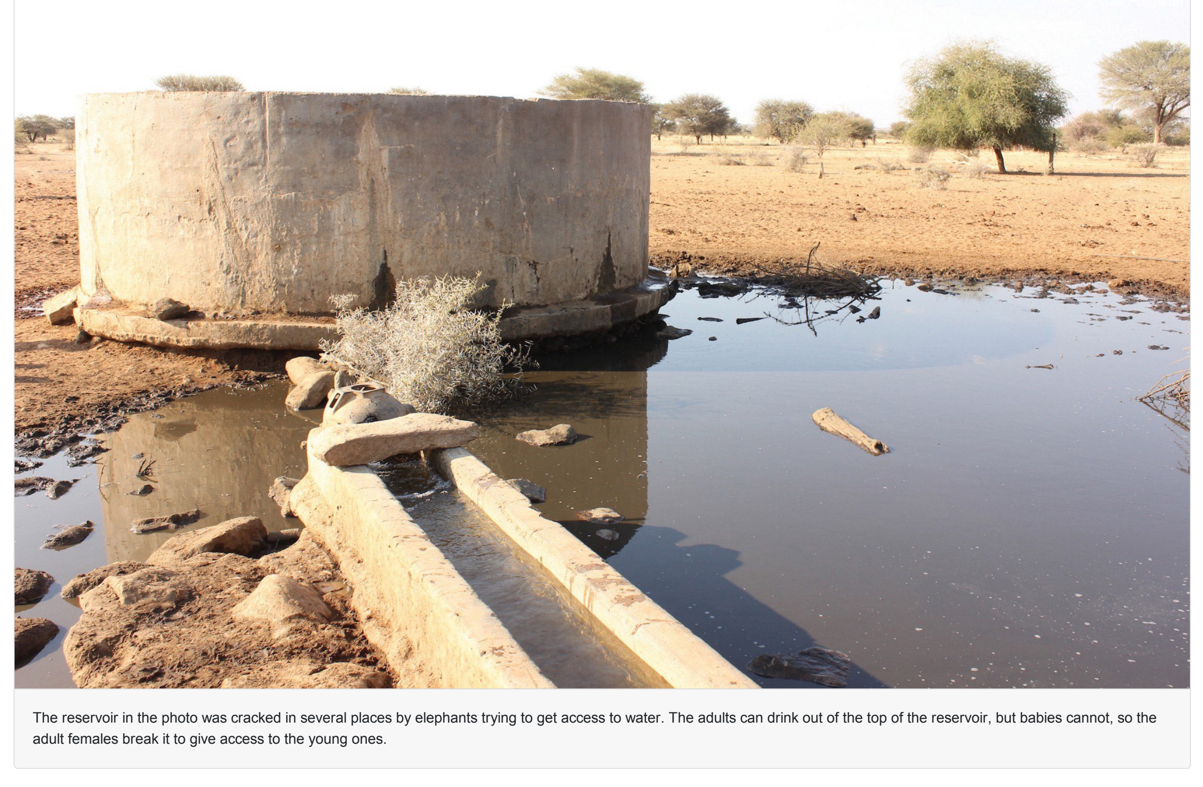
The reservoir in the photo was cracked in several places by elephants trying to get access to water. The adults can drink out of the top of the reservoir, but babies cannot, so the adult females break it to give access to the young ones.
