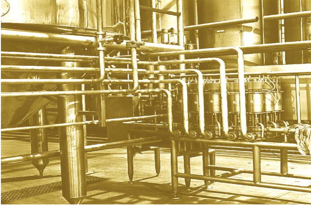
Yeast Propagation Plant. CIP Plant in background
