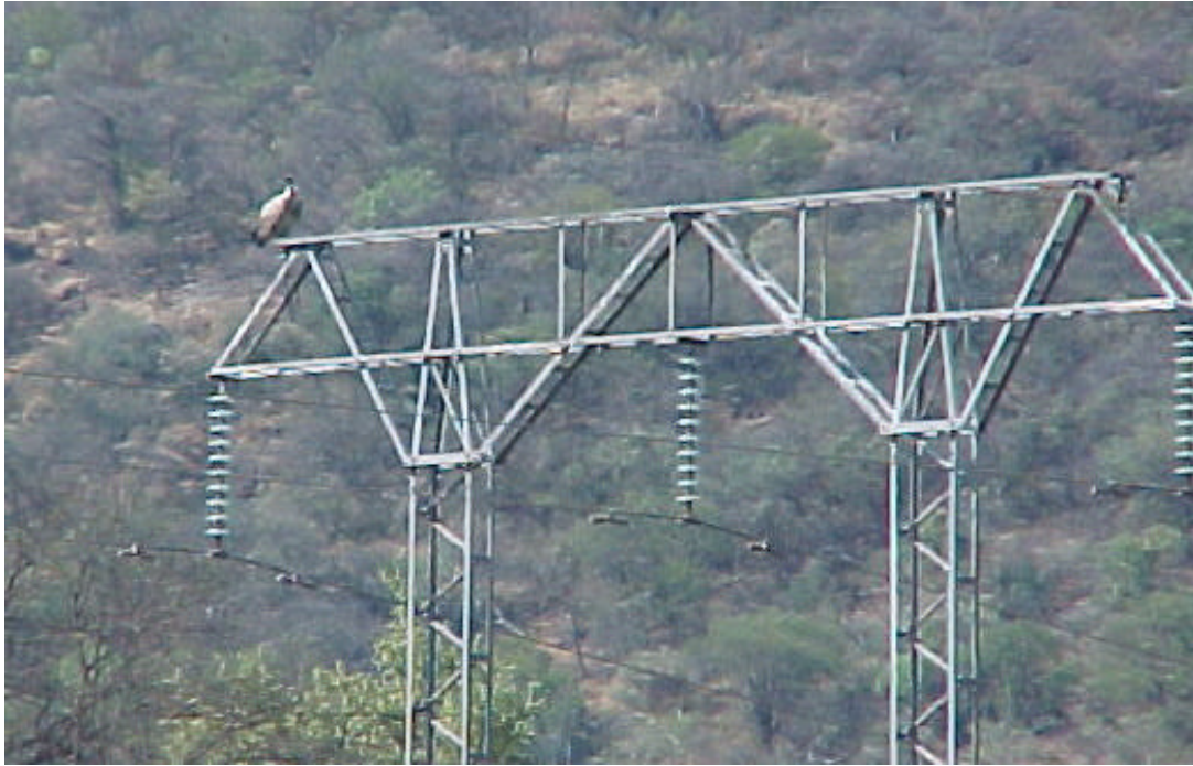
Figure 5. Cape Griffon perched on the Amandel-Thabazimbi Combined 132 kV line.
