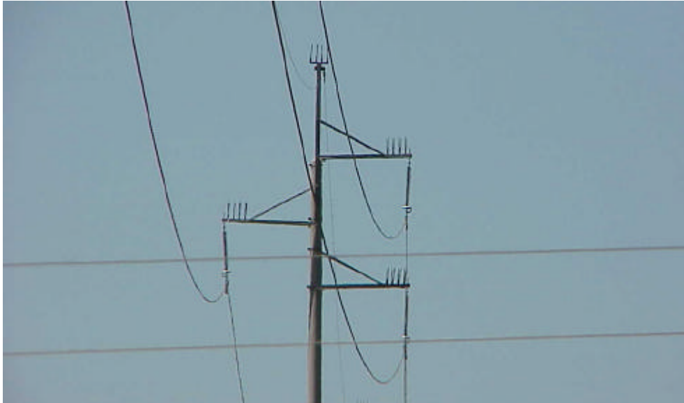
Figure 4. Tabor-Dendron 132 kV line.
