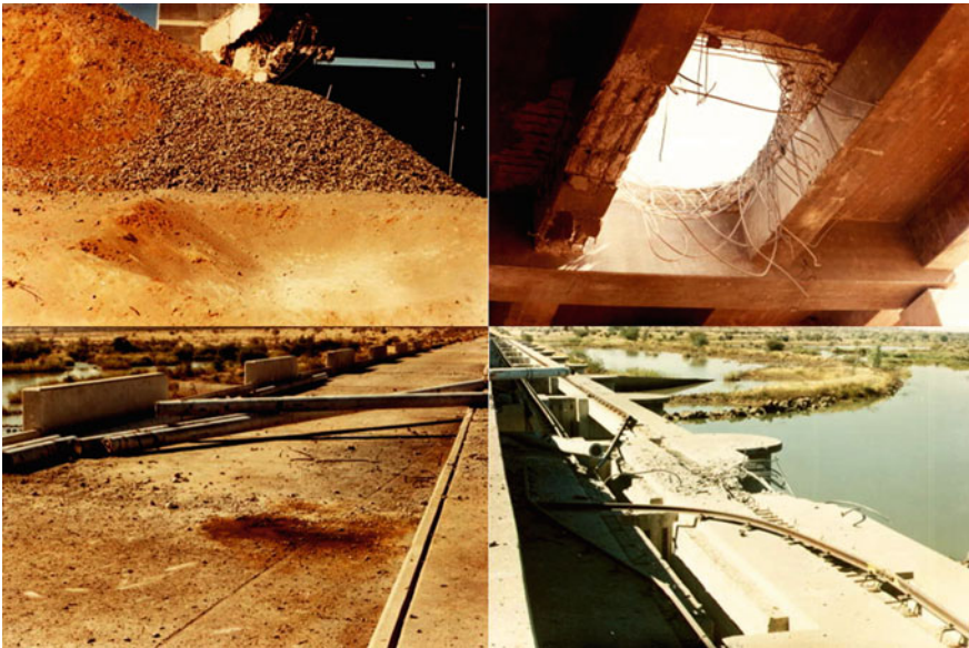
Fig. 2.4 Damage to the Calueque Barrage, June 1988
