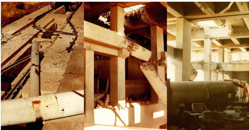
Fig. 2.2 Damage to the Calueque Barrage, June 1988
