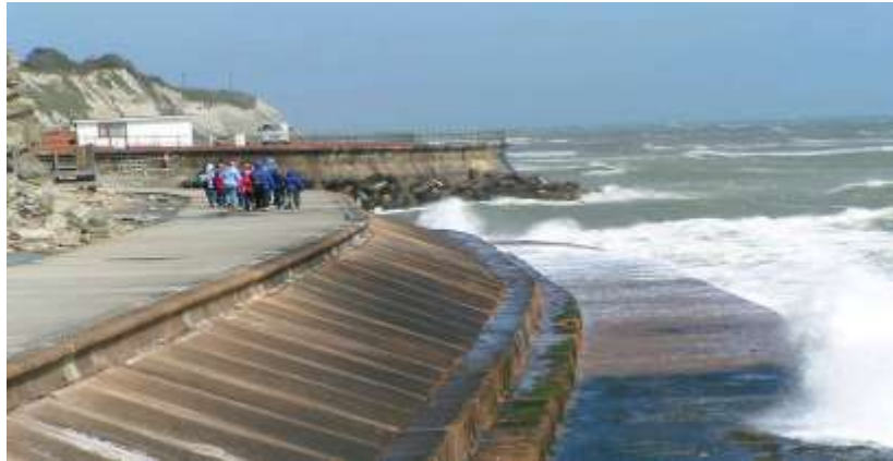
Figure 27: An example of a modern seawall on the Isle of Wight, UK
