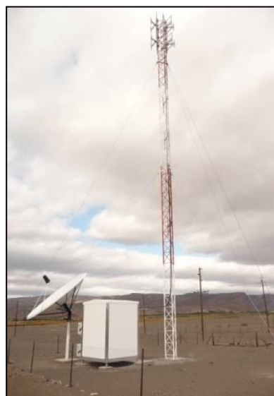
Figure 4: Left: Transmitter tower with antennae
