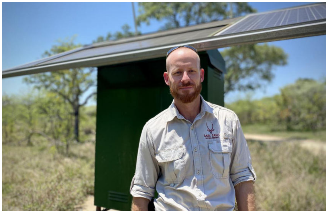
Reserve manager and warden Iain Olivier at one of the reserve’s shock boxes, an installation powered by solar, battery and inverter energy. A single box runs roughly 5 kilometres of fence. The shock box also funnels alarms back to the reserve’s main security control room. (Photo: Tiara Walters)
