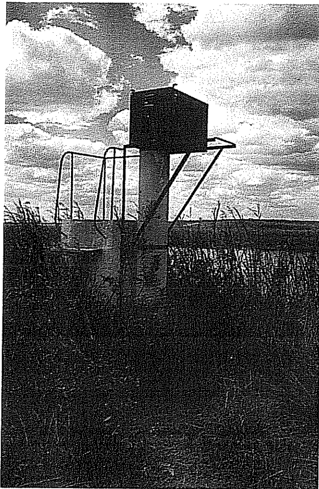
There are broken flow meters at Cuito-Cuanavale and Ciaundo
