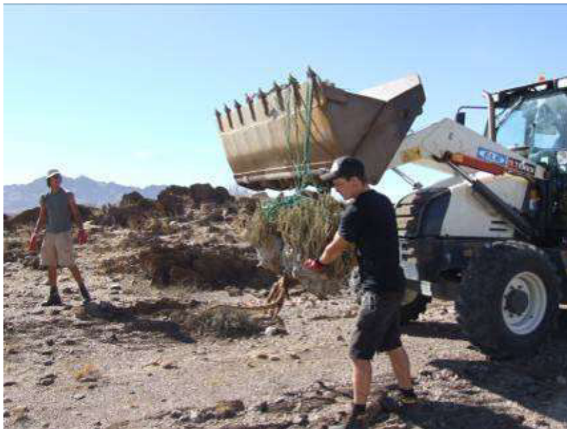
Figure 6. Large plants were fastened with nylon rope and hoisted onto a truck by the excavator (© H. Kolberg).
