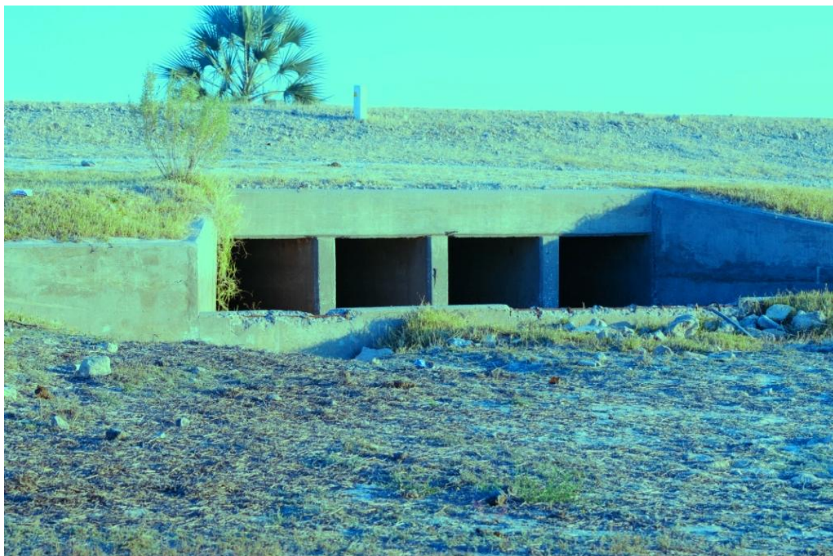
Figure 4-7 Raised floor of bridge over Oshikuku oshana illustrates the raised floor levels of many structures, adding to the flooding risk.
