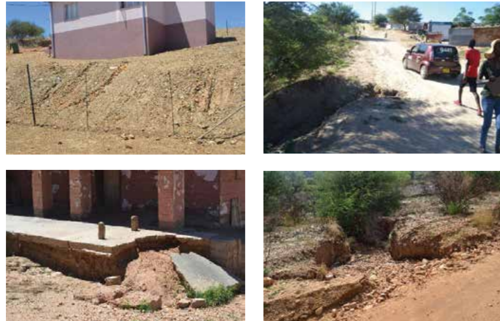
Figure 1: Example of erosion damages to the road and house in Windhoek
