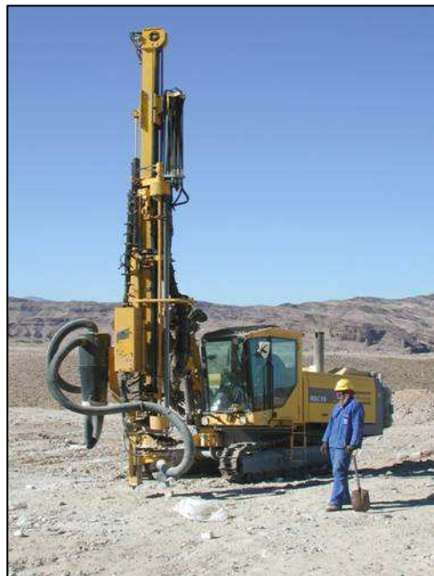
Figure 3.5 Drilling and blasting is sometimes required to break up hard cemented material
