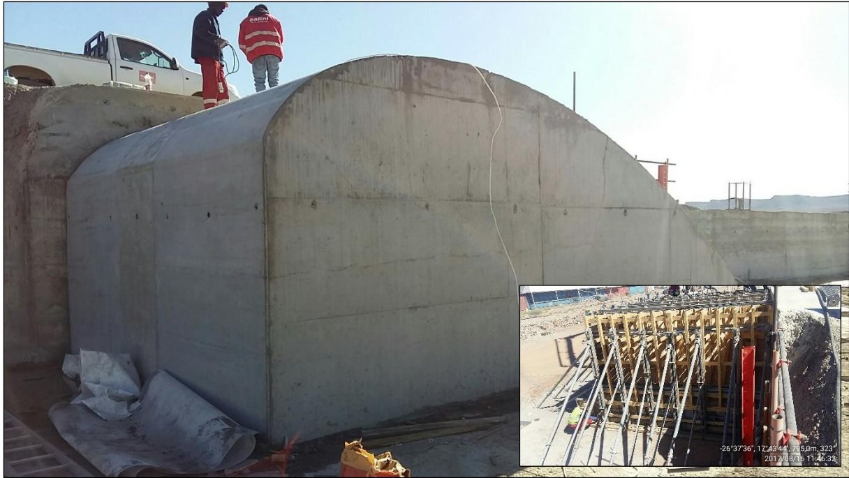
Figure 8. Full-scale Ogee crest trial construction (Insert: formwork erection before concrete placement with CPF liner installed)
