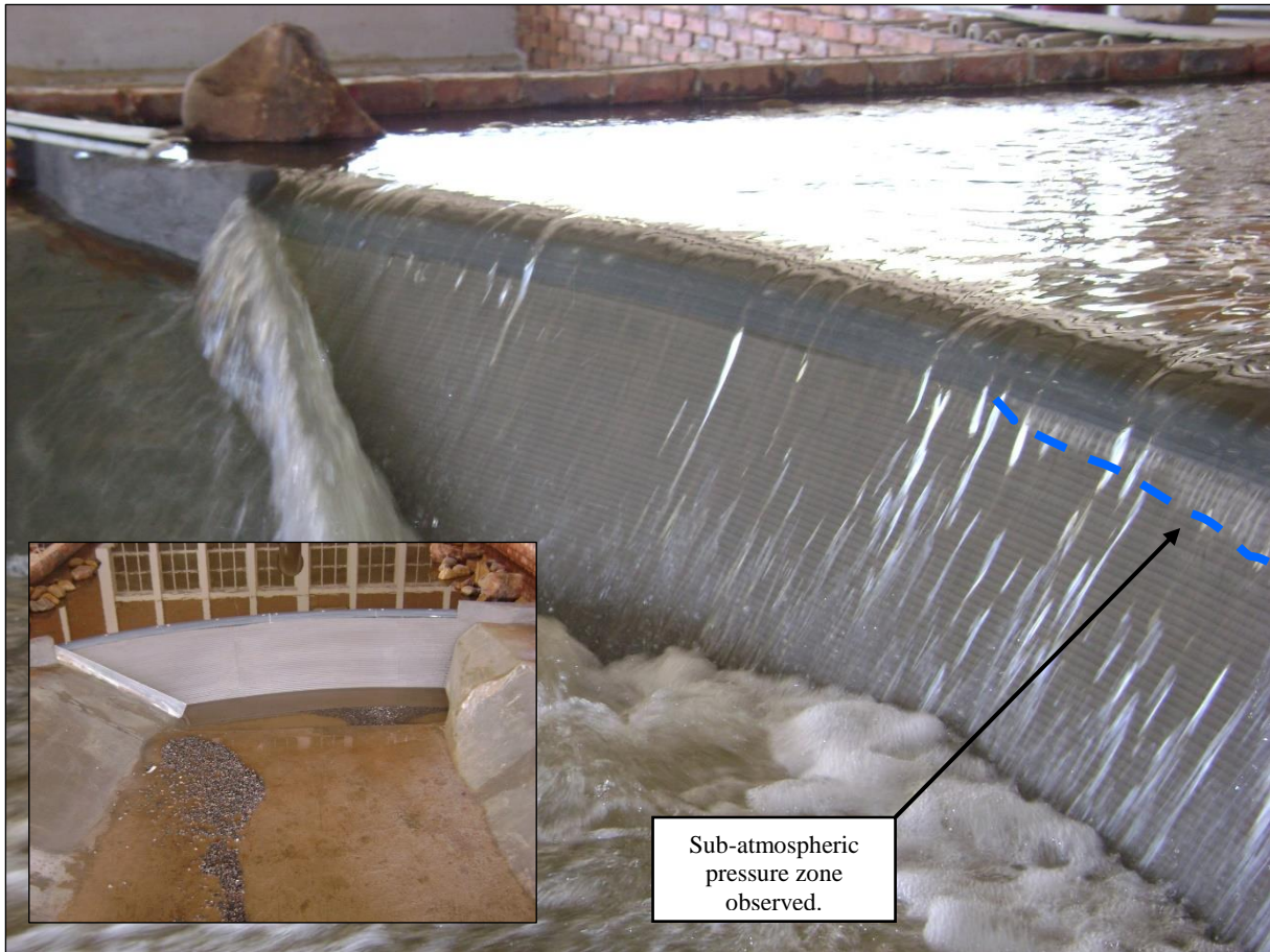
Fig. 4. Flow accentuated towards the downstream wall of the chute. Unacceptable high flow depths were experienced in the chute. Breakaway also observed towards the left bank of the spillway (Insert: Significant erosion and large recirculation flow present during the RDD).
