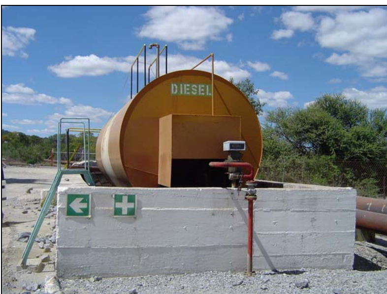
Figure 5.5 An example of an appropriately bunded diesel tank
