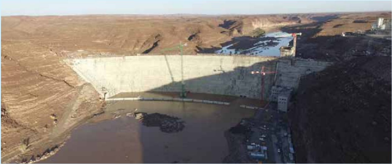
Installation of reinforcements at valve chamber after casting, Abstraction weir, pump station and pipeline
