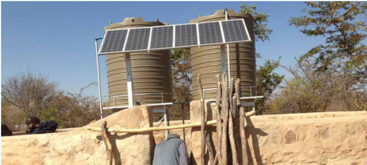
Booster Pump station
