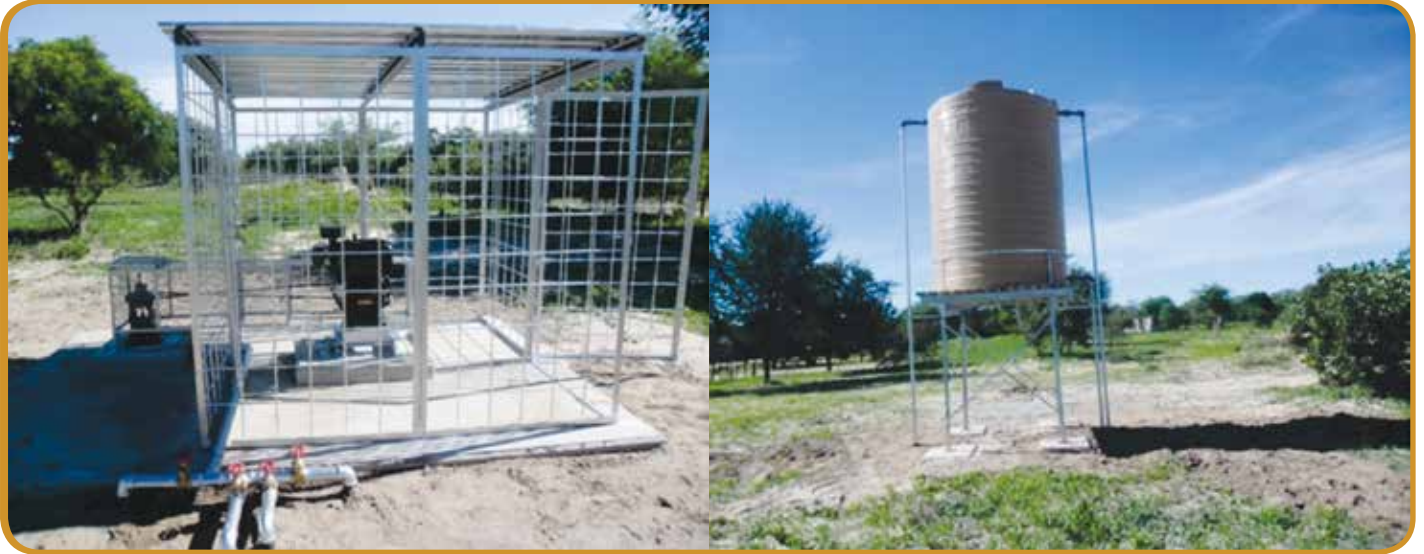
Fig. 1: Water Pump, housepump and water tank installed at Omufitu-Wekuta Community Forest
