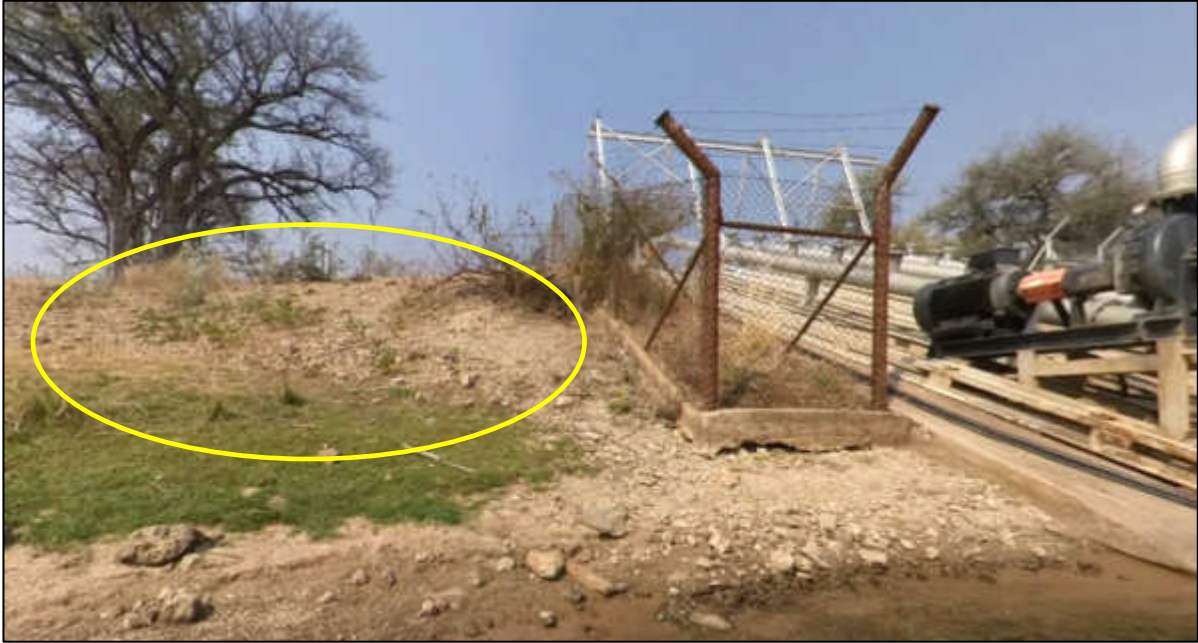
Figure 24: Earthworks to install large abstractions disrupt the soil and natural vegetation creating a window of opportunity for Alien Invasive Plants. Indicated in the yellow circle are Argemone ochroleuca (White Mexican Poppy) and Senna occidentalis (Coffee senna) growing in the disturbed soil alongside an abstraction point – once established these plants will likely spread downstream.
