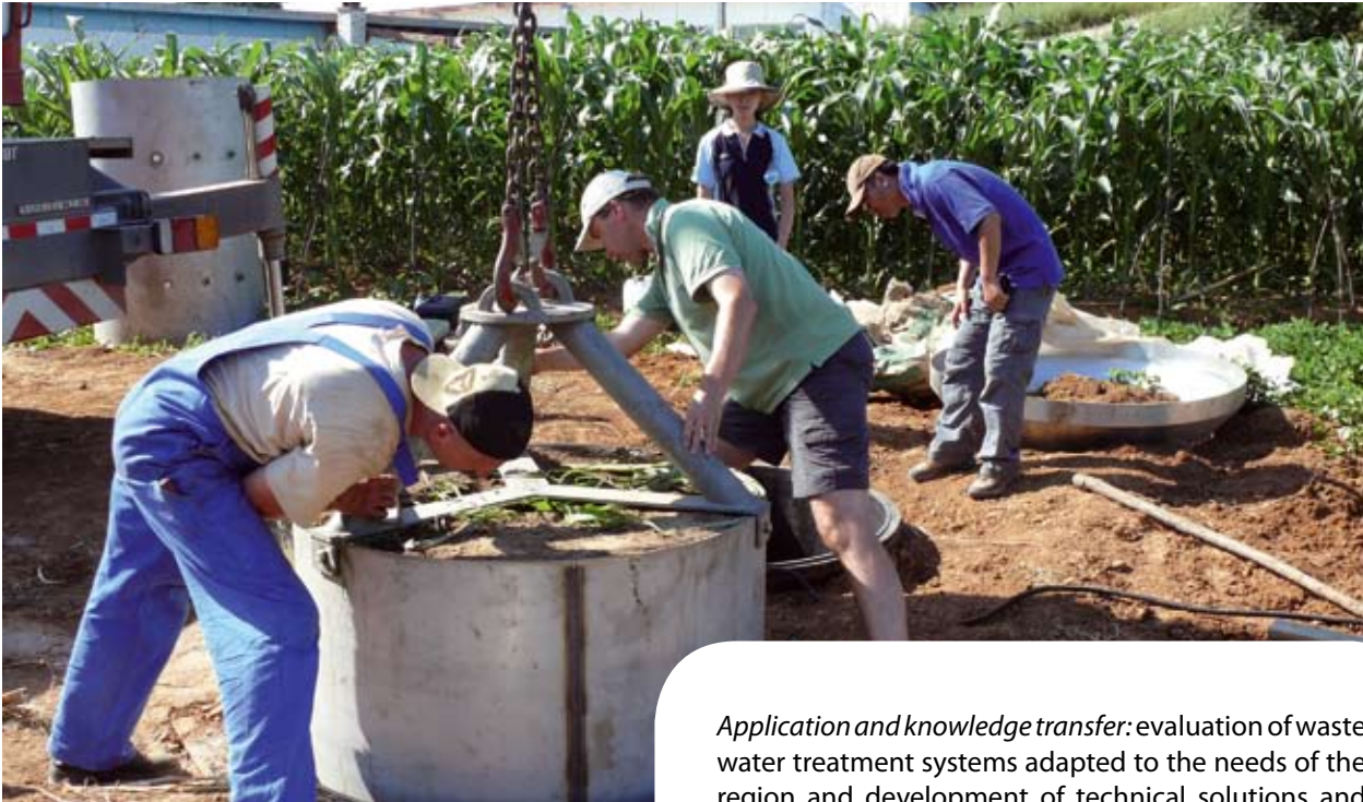
Figure 16: Installation of a sophisticated gravitation lysimeter station (company UGT Muencheberg) at the Shixia research station (Photo: G. Ollesch).
