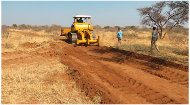
Figure 3: A line is ripped where soil dug from the ditch will be heaped to key in the bund to better secure it with the ground below.
