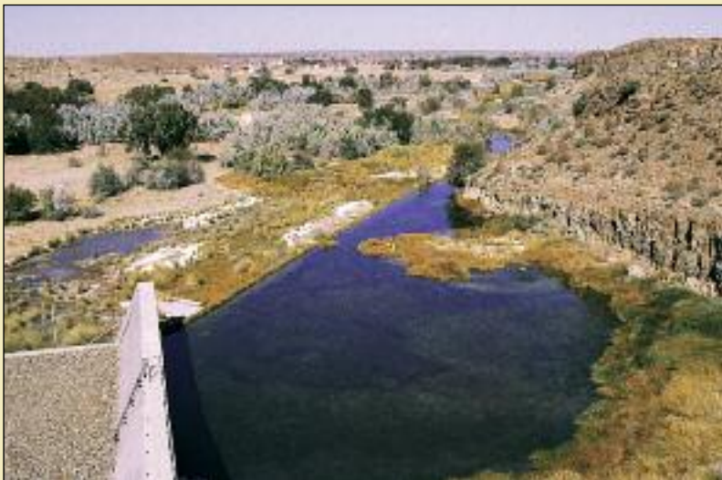
Water seeping through the dam wall of the Dreihuk Dam
