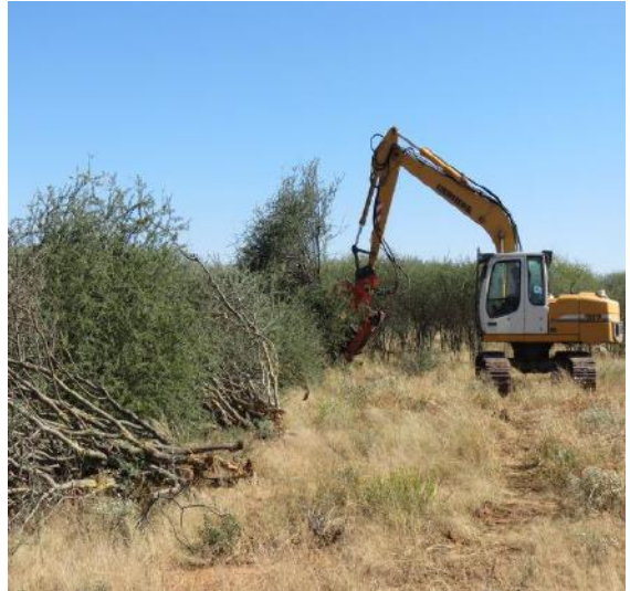
Photograph 7: Windrows being stacked with a hydraulic grab and cutter fitted to an excavator (WoodCo)
